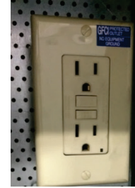
Figure 6 - Field Wired Convenience Outlet
