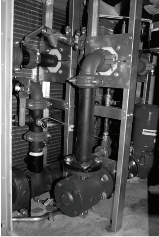
Figure 3 - Heat Exchanger and Pump
