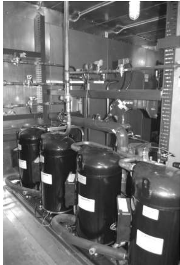
Figure 1 - Walk-in Compressor and Control Compartment
