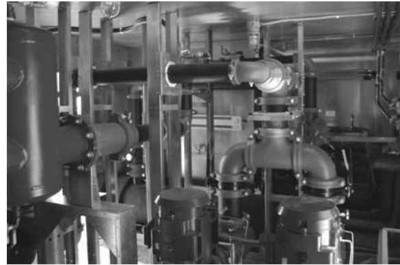
Figure 3 - Chilled Water Pumping Package Piping
