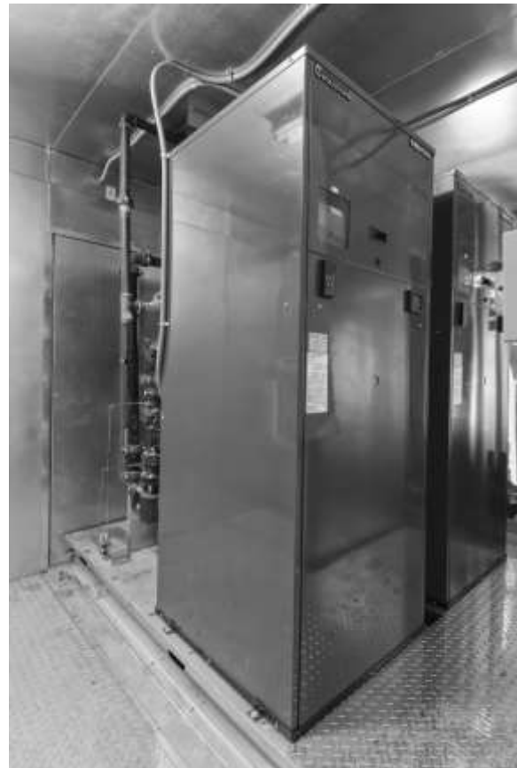
Figure 5 - Factory Installed Boiler
