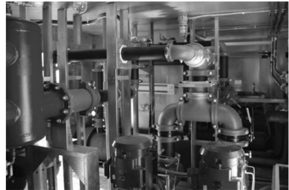
Figure 3 - Chilled Water Pumping Package Piping
