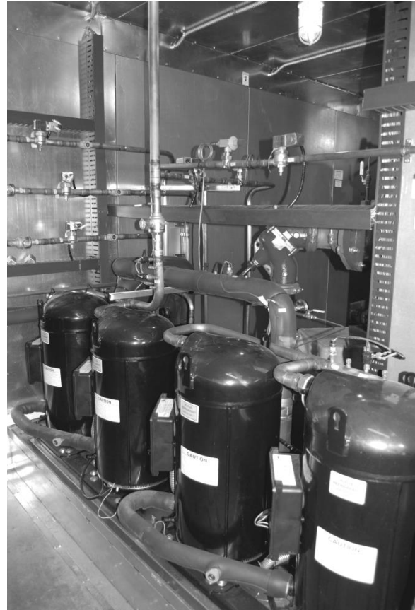
Figure 1 - Walk-in Compressor and Control Compartment
