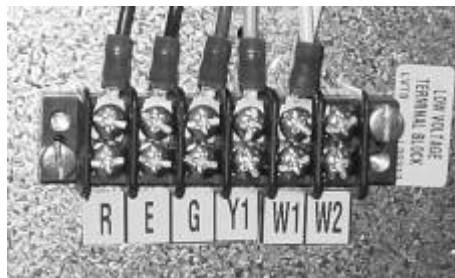
Figure 13 - Example Low Voltage Terminal Block
