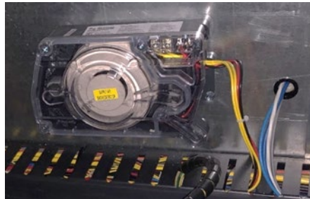
Figure 13: Supply Air Smoke Detector
